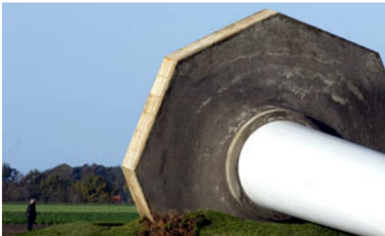
Figure 16. A 70-meter or 230-feet high tower collapsed in inclement weather at Goldenstedt, Germany, on October 28, 2002.
