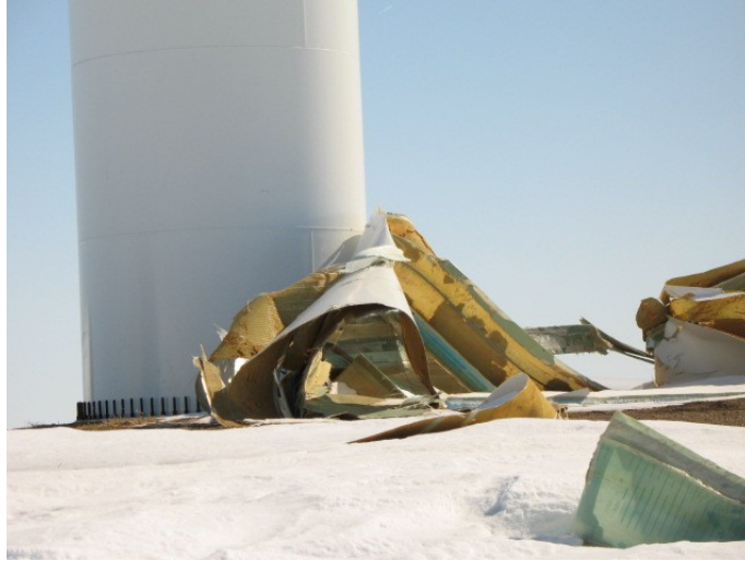
Figure 18. Turbine failure at Lake Wison, Minnesota, November 2007.
