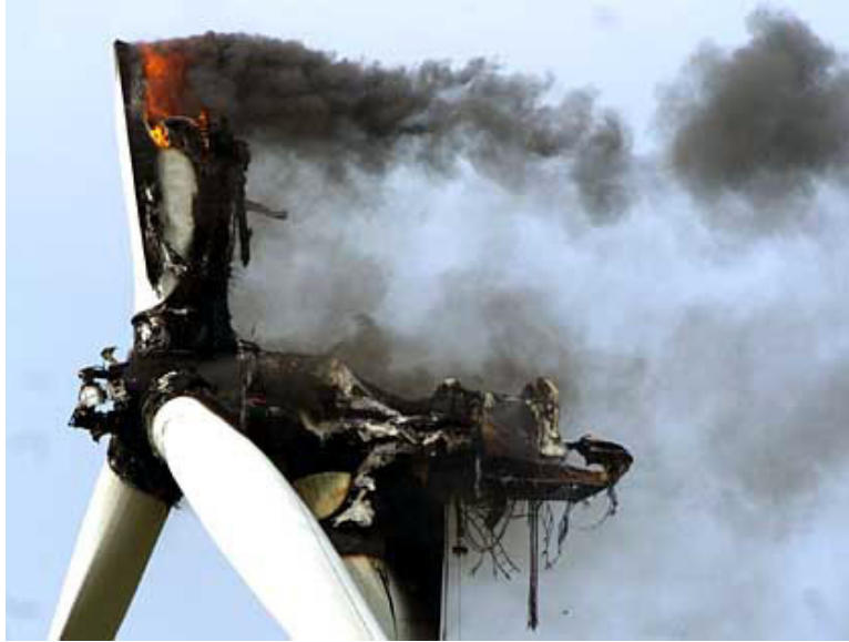
Figure 20. Fire caused by a short circuit, frictional overheating or lightning in 2004 in Germany. Source: Der Spiegel, DPA.
