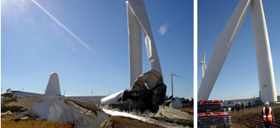
Figure 15. Tower collapse of a wind turbine. Wasco, Oregon, August 27, 2007.
