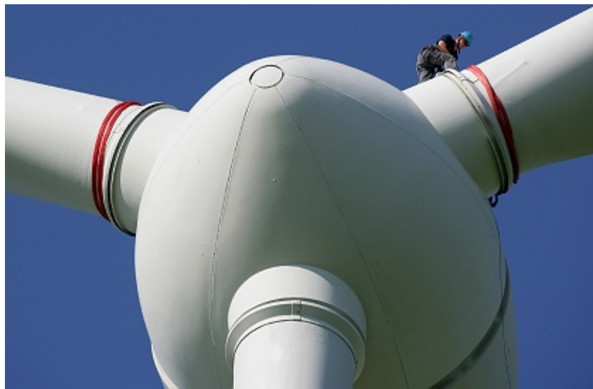
Figure 3. Assembly of wind turbine components entails work at great heights and use of safety harness equipment.
