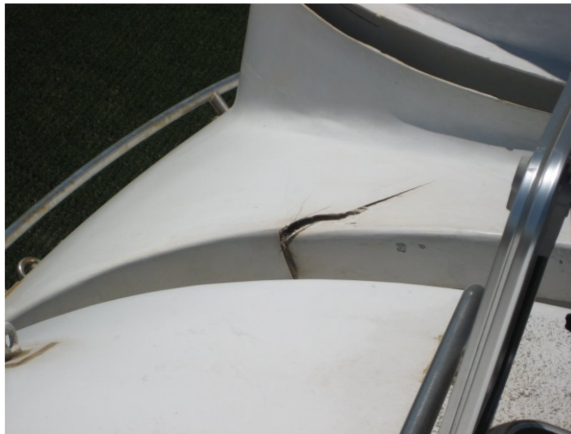
Figure 21. Structural crack near the hub of a wind turbine.
