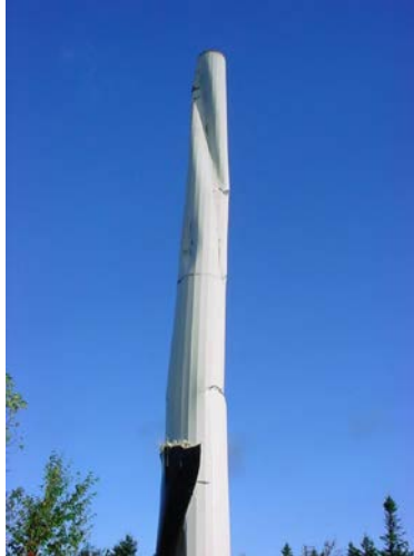
Figure 10. Turbine collapse in high wind conditions at the Searsburg, Vermont wind facility, September 15, 2008.
